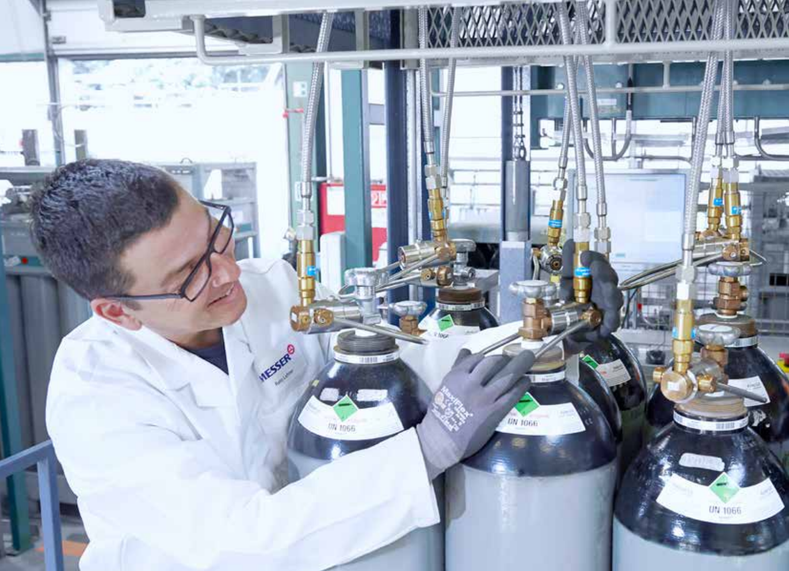
Filling station for high-purity gases in Lenzburg
