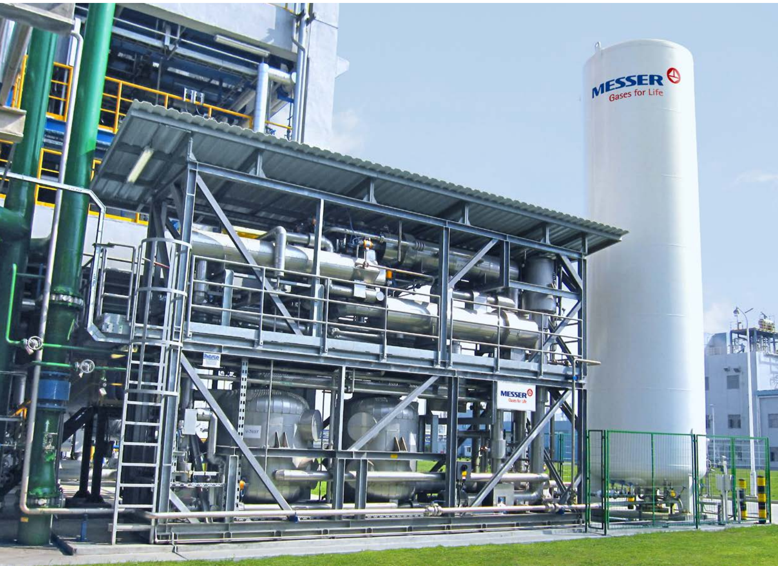
Recovery unit for methyl chloride
